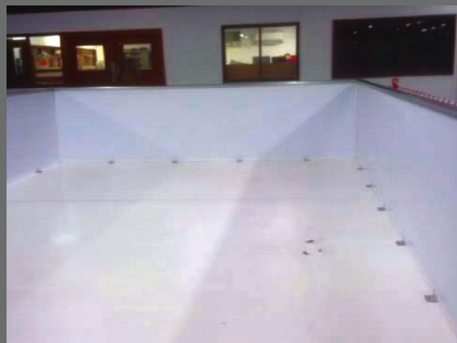
Free-standing low level hoarding
